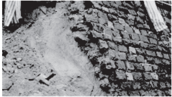
Figure 14. Close view of the collapsed retaining wall
