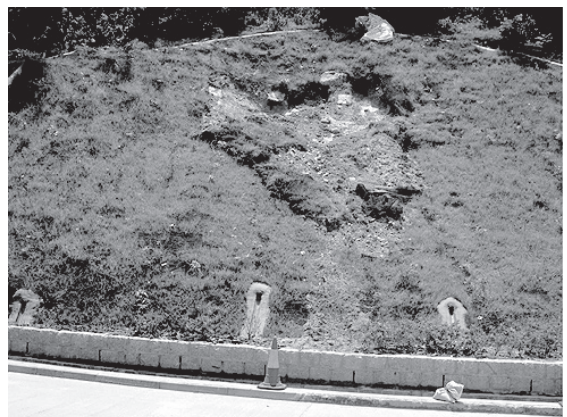
Figure 22. Local failure at a soil-nailed slope
